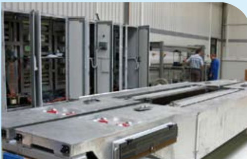
eMASS at HySCO (CGL) in Dangjiin, South Korea with adapted carrier construction
