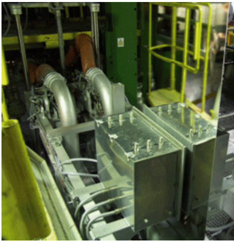
Fig. 1: Installation of an eMASS system above the air knives in a hot dip galvanizing line
